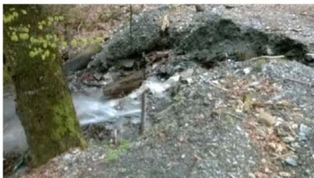
DAMAGE DETECTED BY FLOW METER DIFFICULT TO ACOUSTIC DETECT
