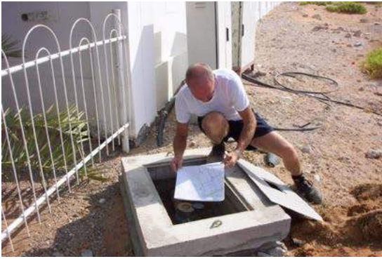
Leak on a service connection identified through a visual inspection of the system
