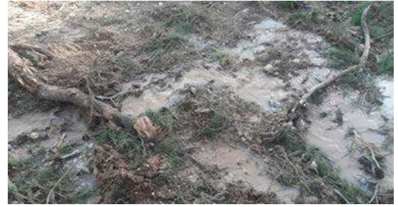
Eventually, the main leak was found in a natural creek outside the residential area. Without TaKaDu, the leak would probably not have been discovered for another 6-10 months.
